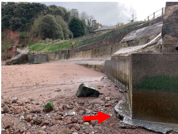
No AIMS Asset ID Low beach levels and undermining of toe.
