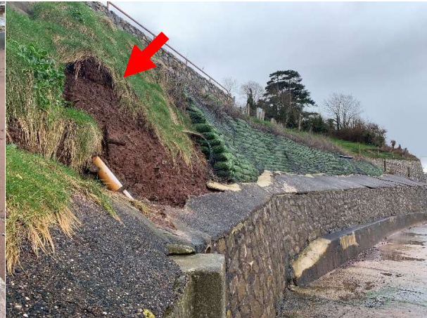
No AIMS Asset ID Erosion of grass bank as southern end of wall.
