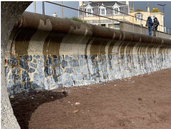
177501 Upper concrete bullnose and masonry facing in good condition, high beach levels.
