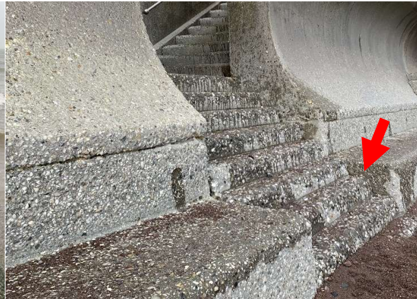
177697 Heavy abrasion of concrete toe and steps.
