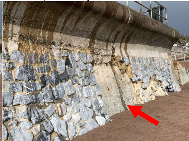
177501 Localised loss of section of masonry facing at northern end of wall exposing concrete backing.
