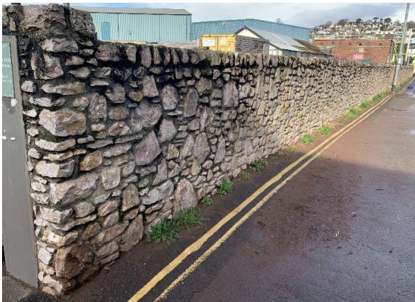
180688 No gaps or cracks in masonry or mortar joints in new walls constructed.
