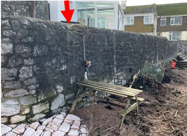
392776 Masonry blocks and mortar joints good, two short sections of missing coping stones.
