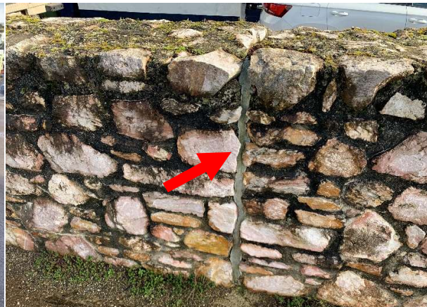
180688 Joint sealant in new masonry walls remains in good condition with no signs of debonding or cracking.
