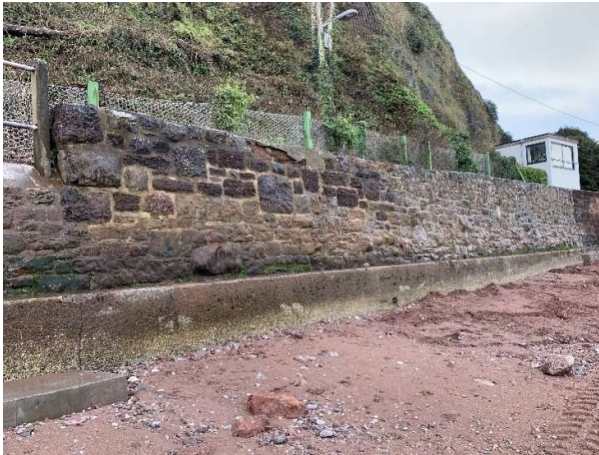
84538 Masonry blocks generally in good condition with no cracks or gaps in mortar.
