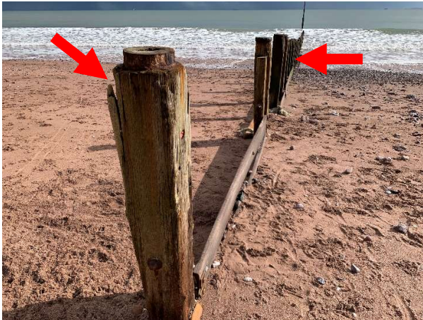
327084 Most posts vertical with only minor rotation evident. Many posts split and cracked.
