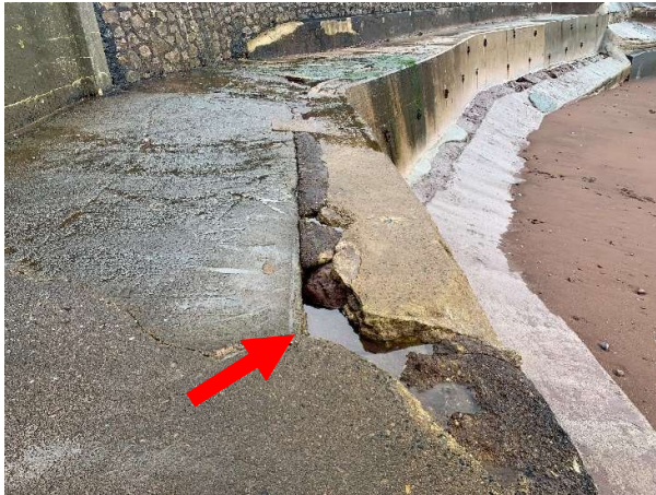
No AIMS Asset ID Cracks in concrete and rendering, some sections of concrete broken and missing.
