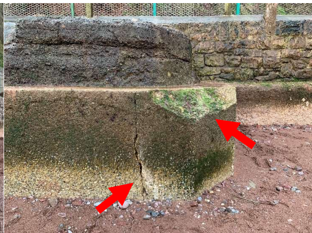
84539 Abrasion along concrete toe and localised cracks and missing sections of some concrete.
