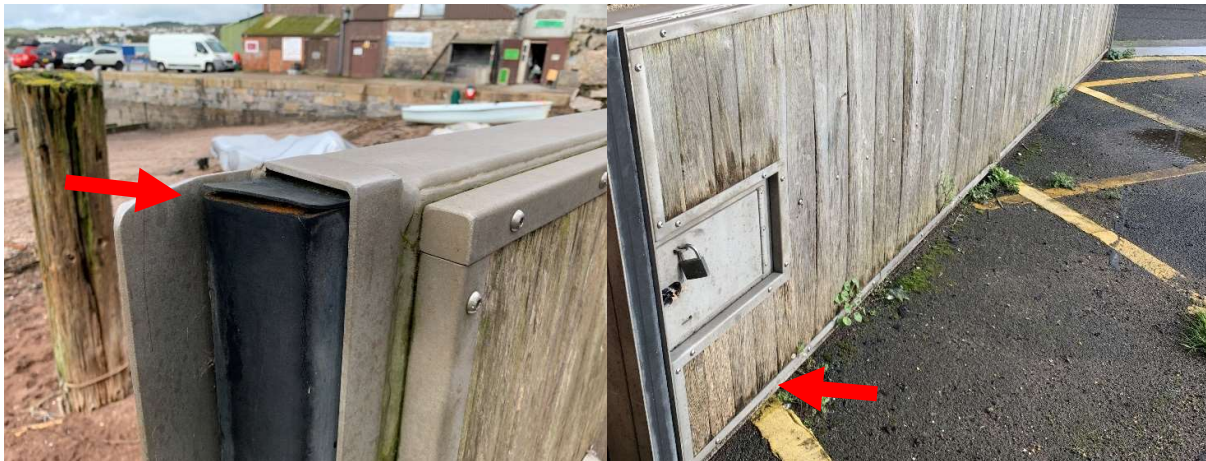
392754 Minor cracking evident to most rubber seals, with some delamination of one seal (flood gate No.12).
