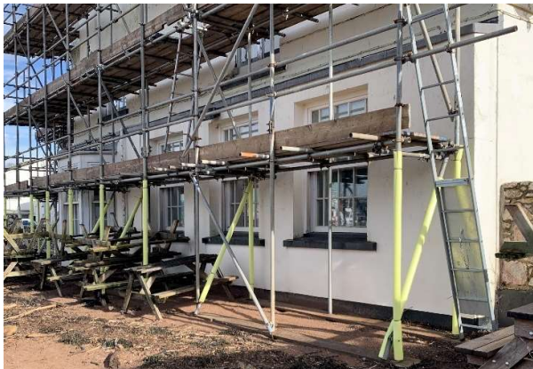
392734 Property wall of the New Quay Public House in good condition, windows do not appear to be floodproof.
