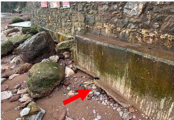
84537 Low beach levels at southern end of wall near outfall resulting in localised undermining up to 0.9m deep.
