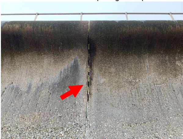
177697 Loss of expansion joint sealant at most joints.
