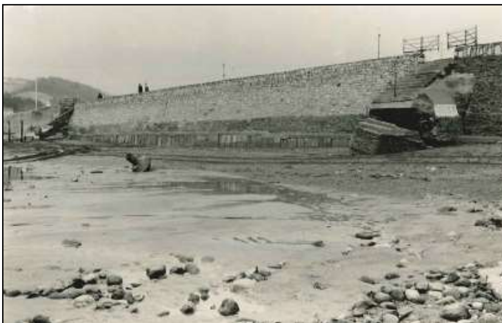
Figure 2.5 Low beach levels between groyne 12 and 13 in December 1975 allowed exposure of concrete piles at the base of the seawall (Gundry, 1982).
