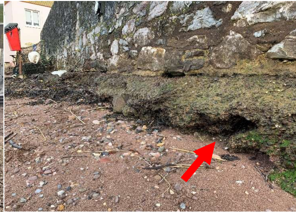
Evidence of beach lowering and some undermining of toe of masonry boundary wall.
