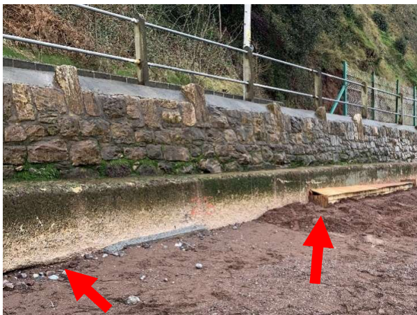
84539 Evidence of undermining of concrete toe, concrete fill repairs underway at time of inspection.
