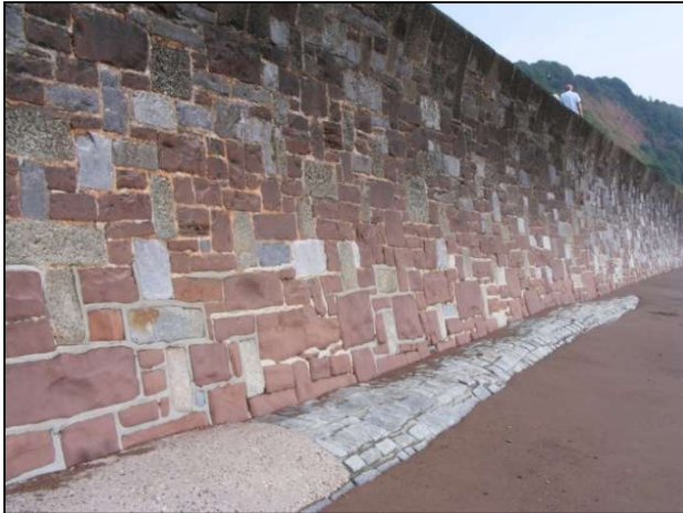
Figure 2.15 Defence protecting the railway line between Sprey Point and East Cliff.
