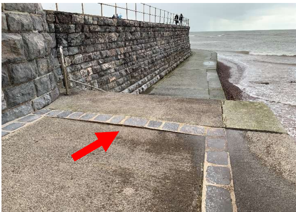
57776 Lifting of areas of infill masonry in between concrete slabs.
