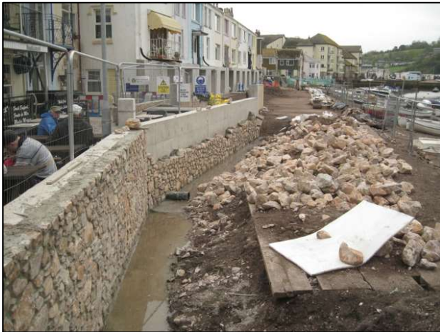
Figure 2.17 Construction of reinforced concrete flood walls with masonry facing as part of the Teignmouth flood defence scheme (R. Scott 2012).
