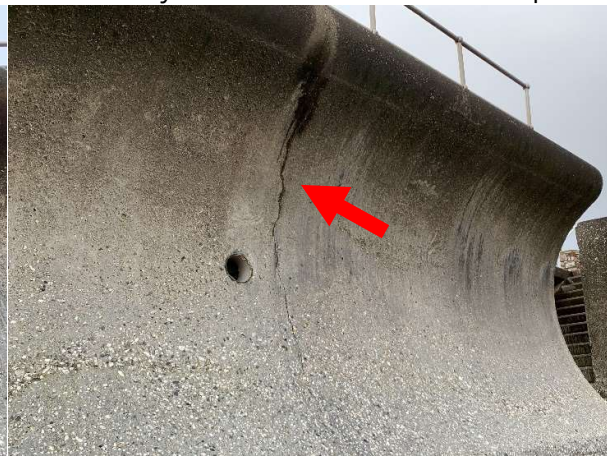
177697 Vertical cracks in upper recurved section of wall at mid-point of many wall sections.
