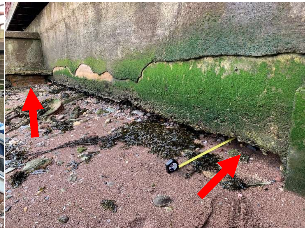
3934 Some cracking and spalling evident in concrete render, beach lowering and localised undermining of toe.
