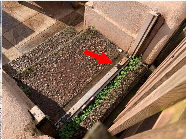
332936 Some loss of paint to aluminium channels for flood boards.
